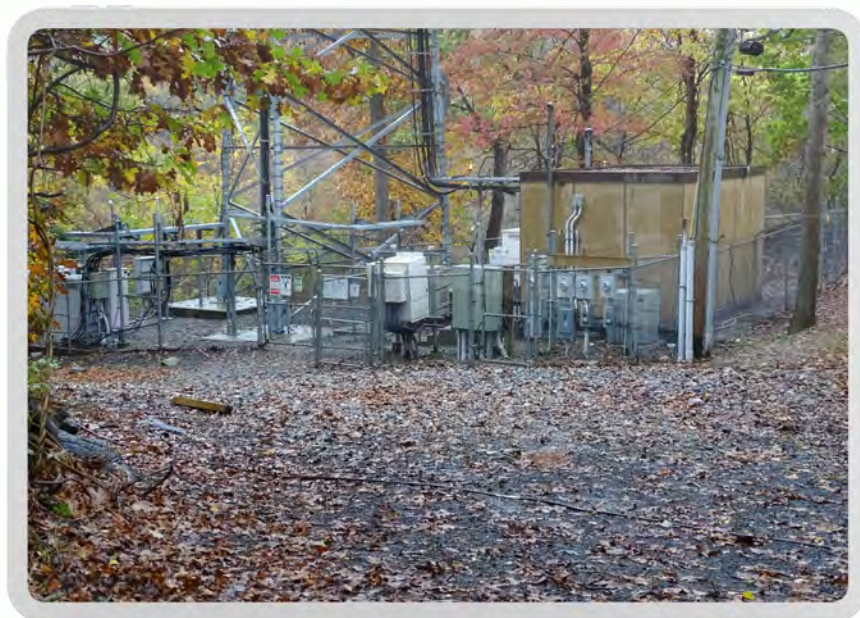
Site Y14 Ground Equipment
