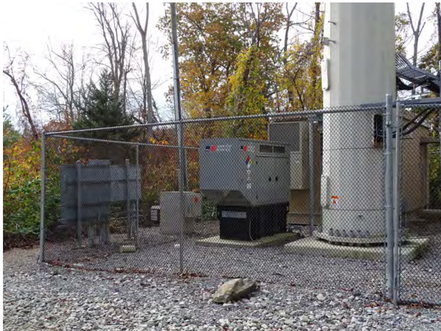
Generator at Site L1
